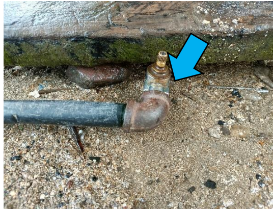
Figure 5. There was no oil contamination in the freshwater used in the households since water comes directly from the mountain, with pipes (blue arrow) found throughout the community.
